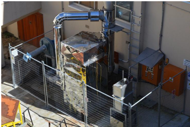
Fig. 1 Packed bed thermal storage facility
