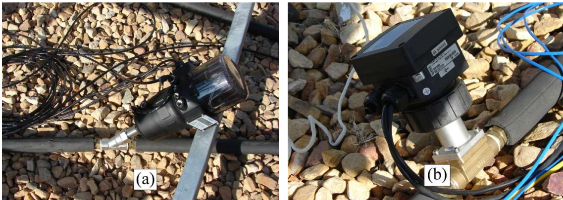
Fig. 7. Angle seat valve (a) and electromagnetic flow meter (b)
