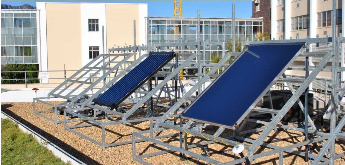
Fig. 9. The reference and client collectors undergoing testing
